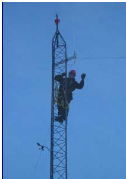
ET3 Frank Tobar putting the up 130 foot tall all band HF Windom
